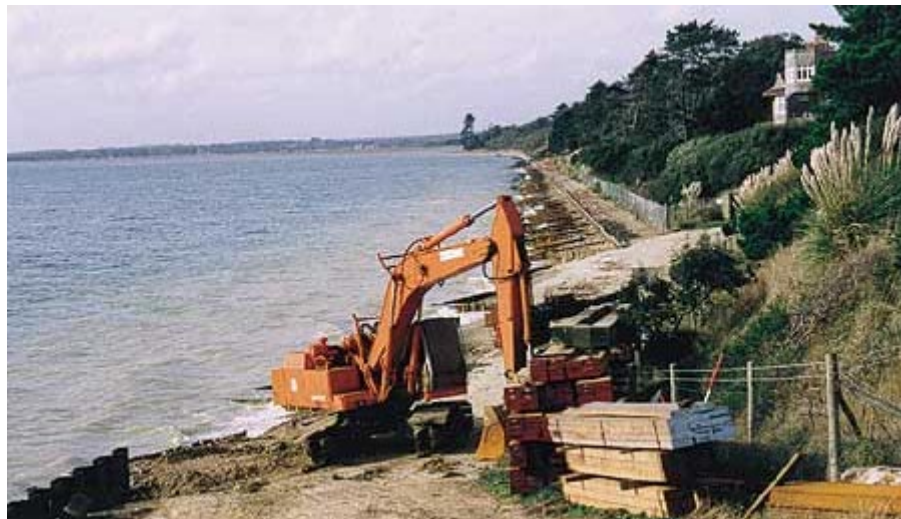
Plate P7b Heavy machinery engaged in coastal defence works west of Lepe proffers an opportunity to examine the stratigraphy of this ancient shoreline at the mouth of the Beaulieu River
